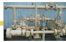
Stop #3 30 psig typical Sampling & Regulator Station
