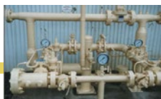
Stop #5 30 psig typical Industrial User Transfer Station
